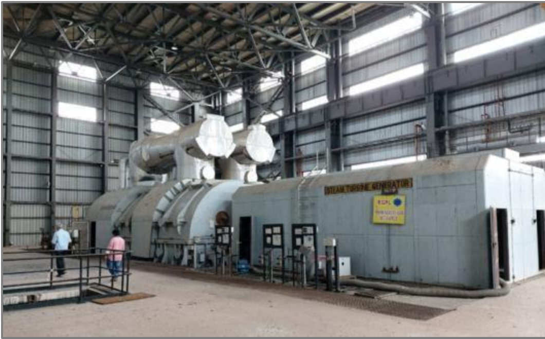
Steam Turbine & Generator
