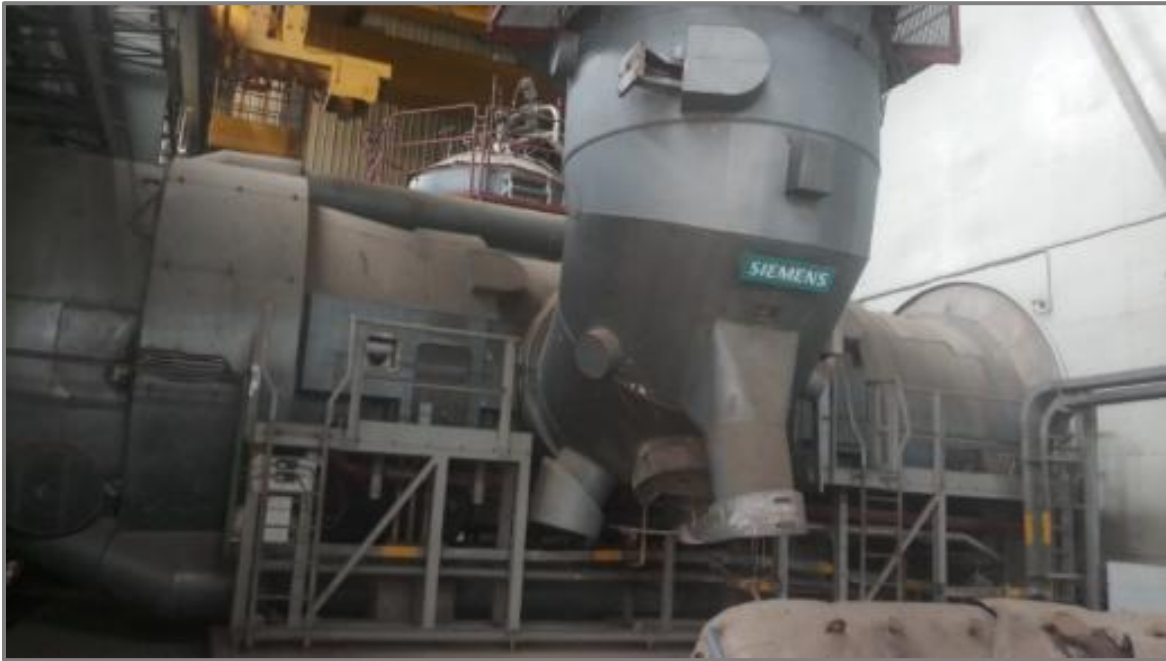
Gas Turbine GT# 1B
