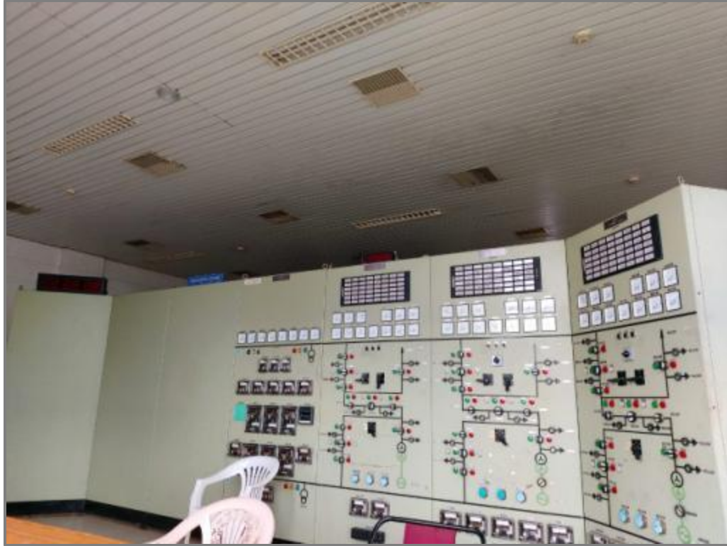
Switch yard Control
