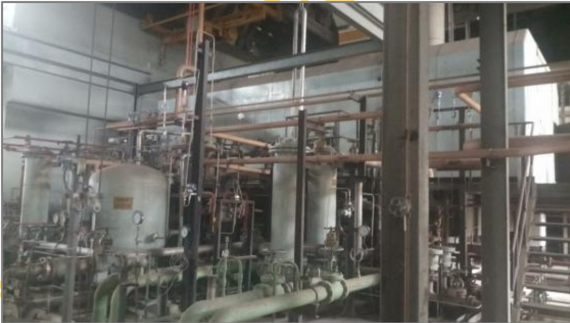
Gas Turbine Generator & Auxiliaries
