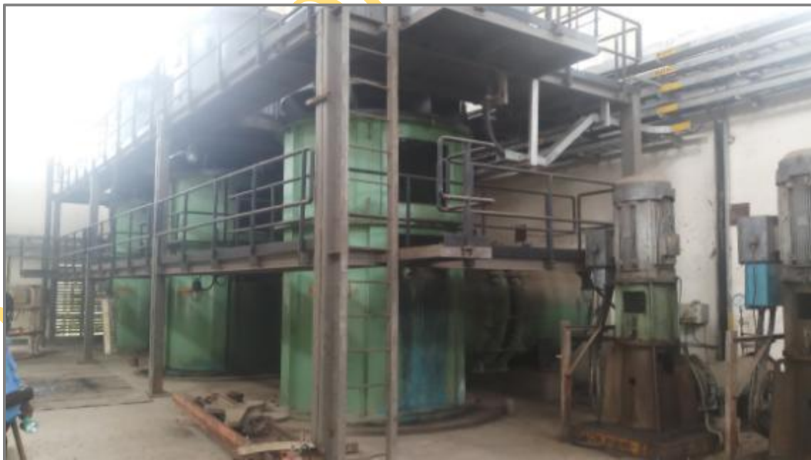
Cooling Water Pumps
