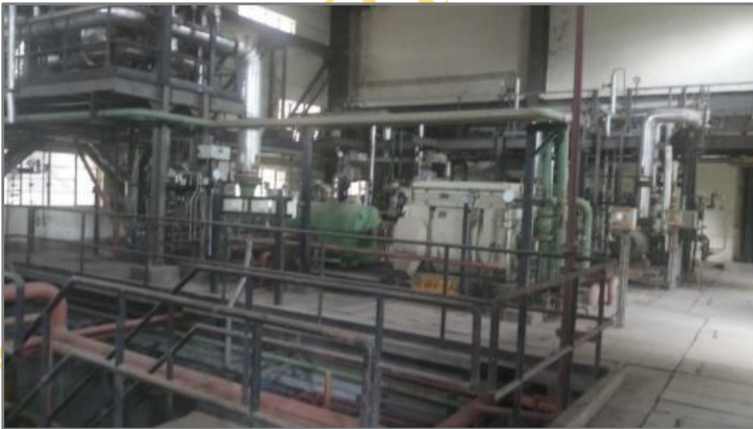
Steam Turbine Auxiliaries
