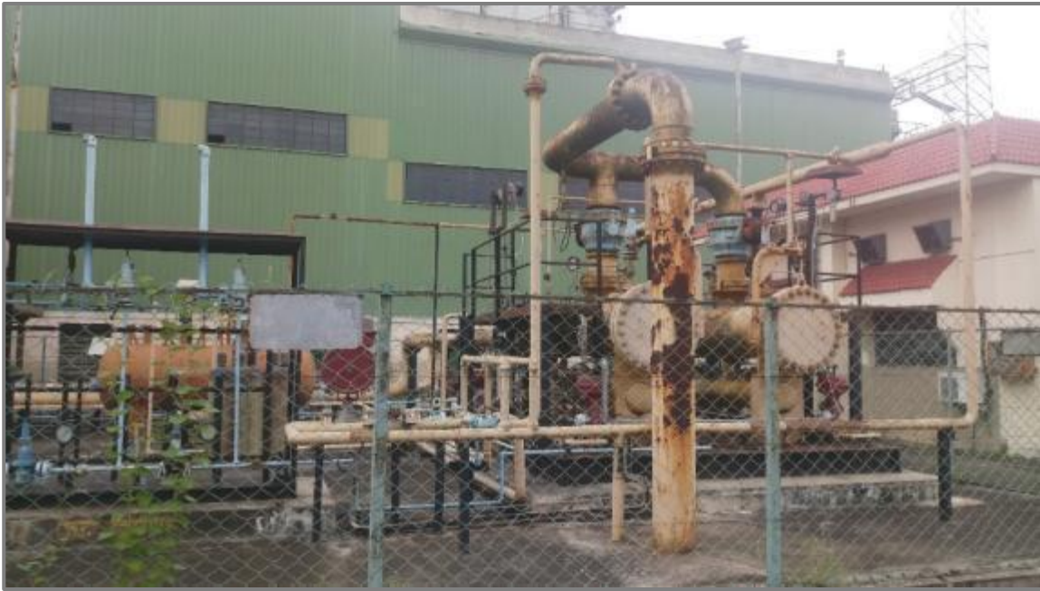
Gas Conditioning Skid
