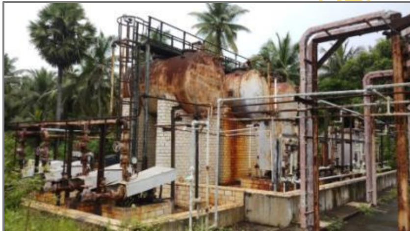
Tanks for DM plant
