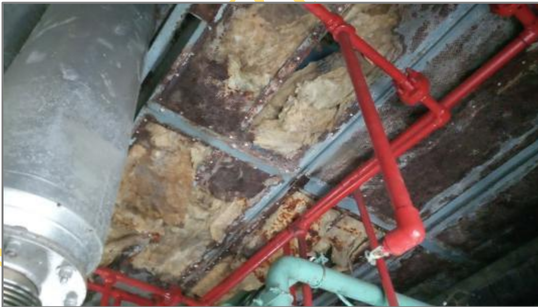
Top enclosure of DG Set
