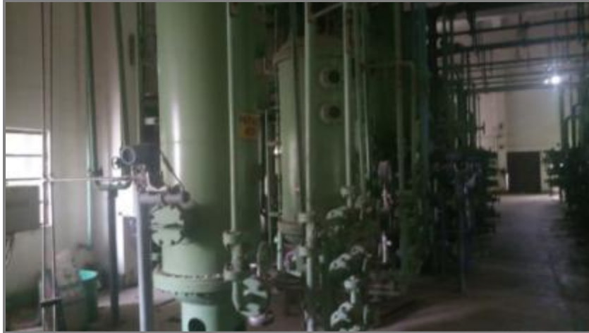
DM Water Plant
