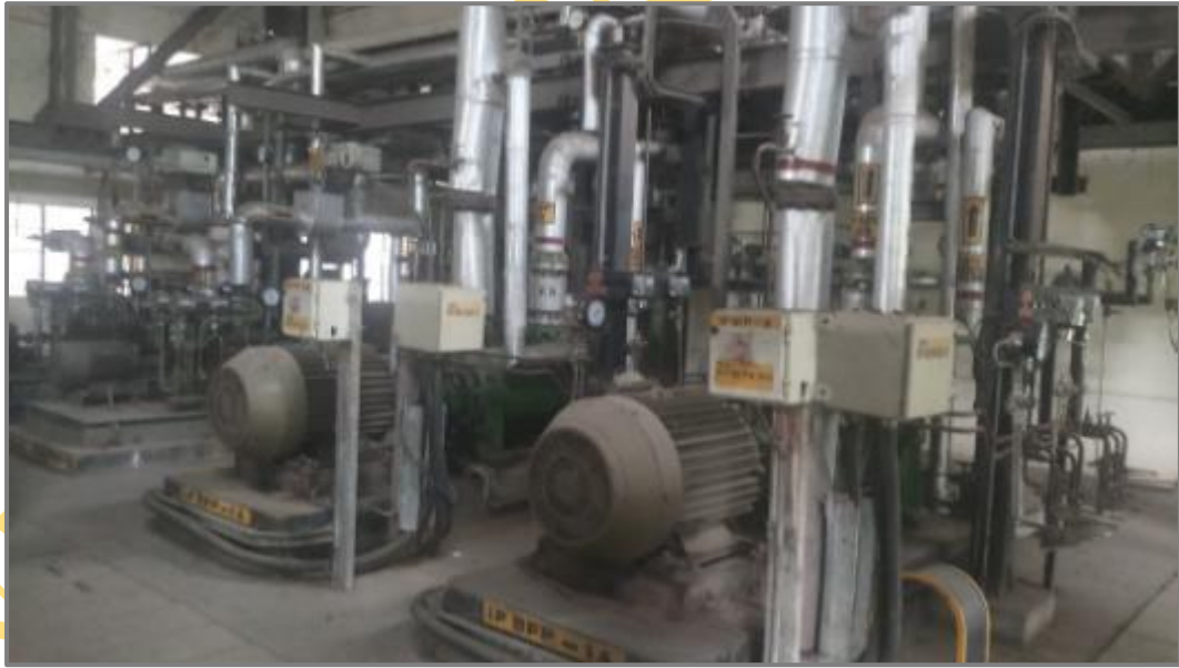
Condition of IP Boiler Feed Pumps
