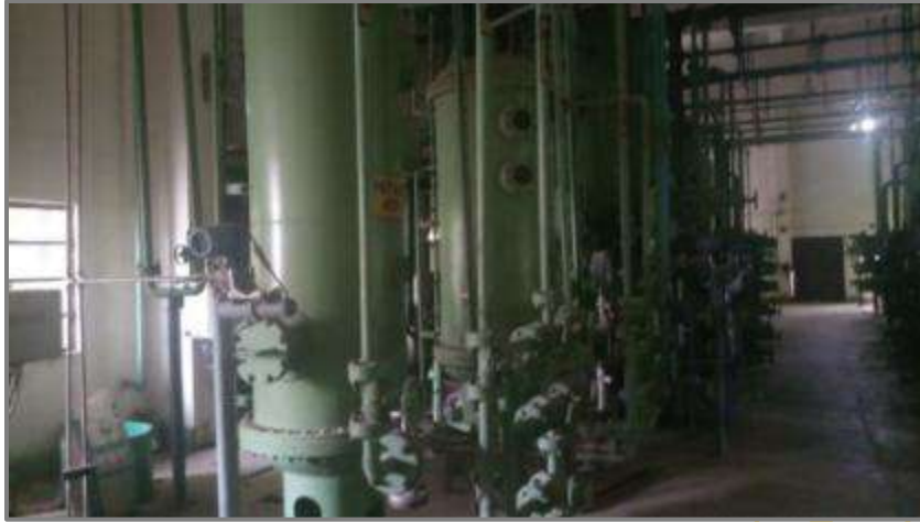
DM Water Plant
