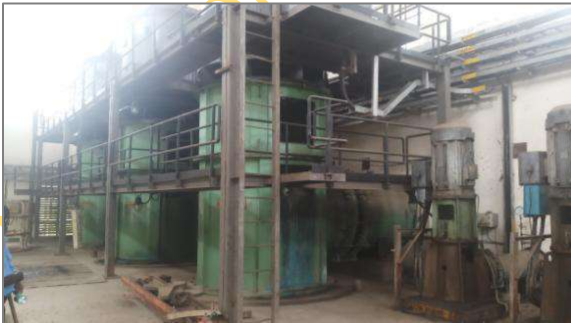
Cooling Water Pumps
