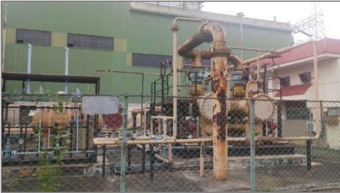
Gas Conditioning Skid
