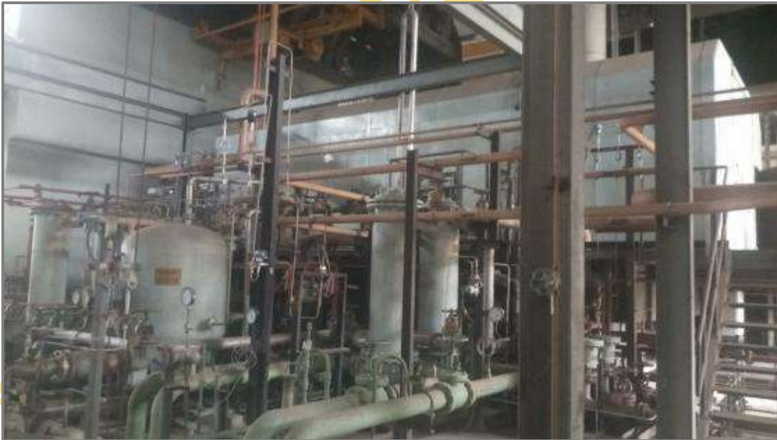
Gas Turbine Generator & Auxiliaries
