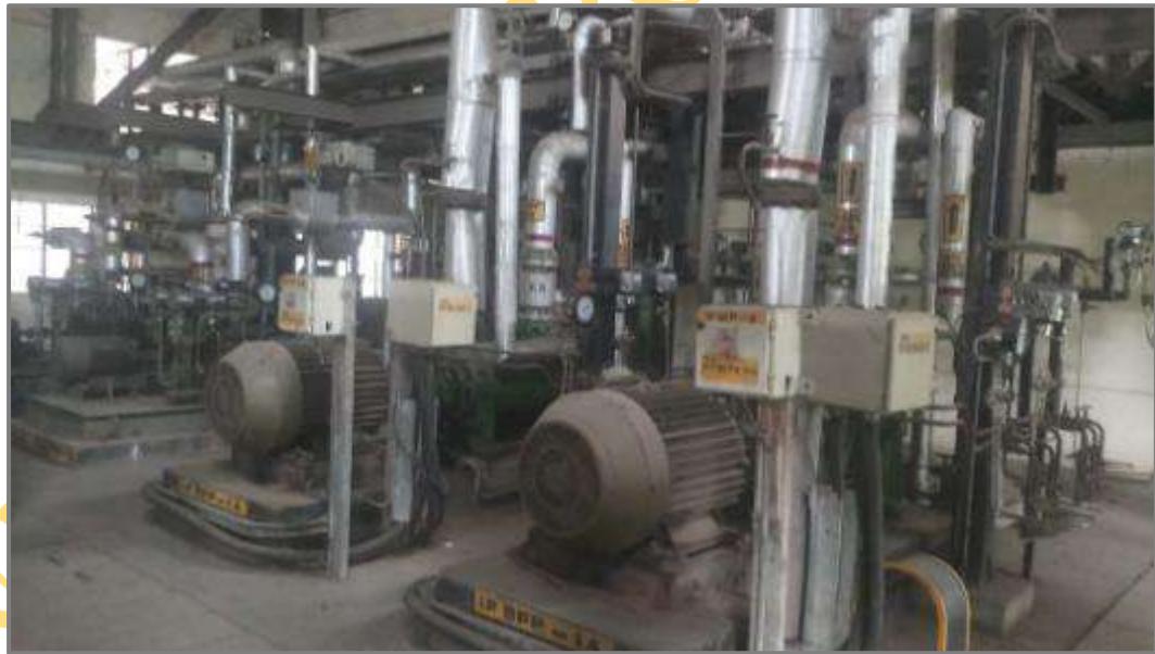
Condition of IP Boiler Feed Pumps
