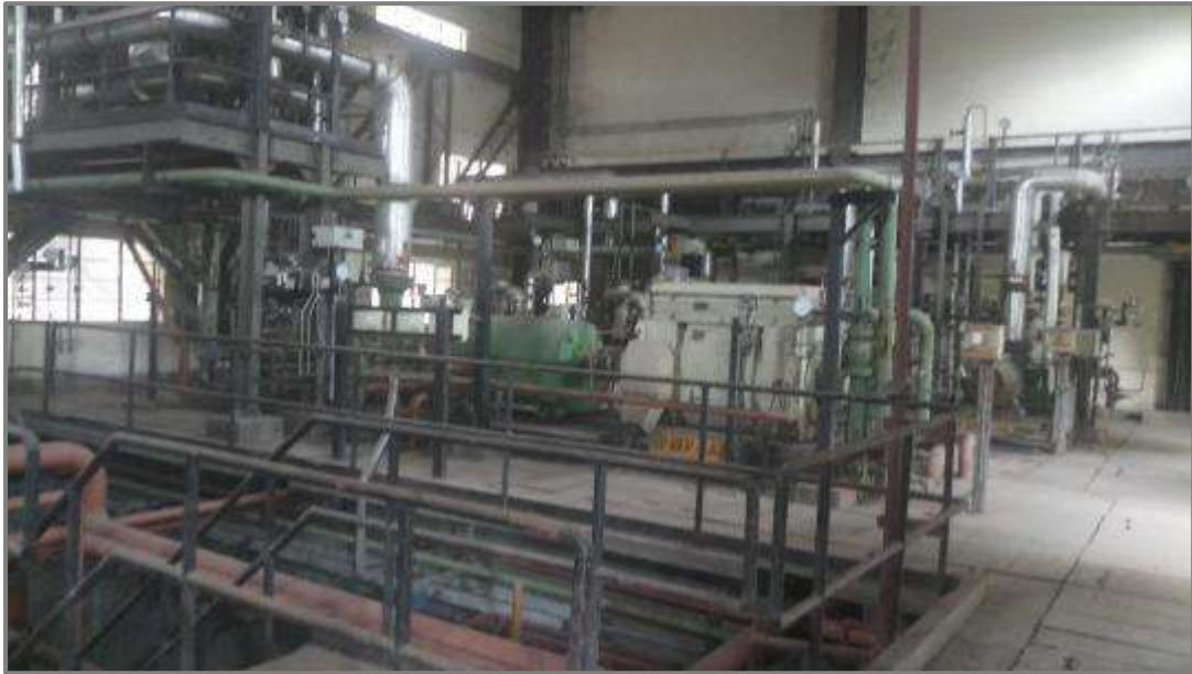
Condition of HP Boiler Feed Pumps
