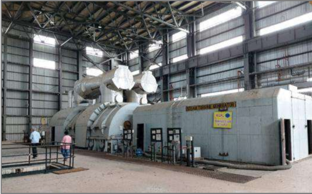
Steam Turbine & Generator
