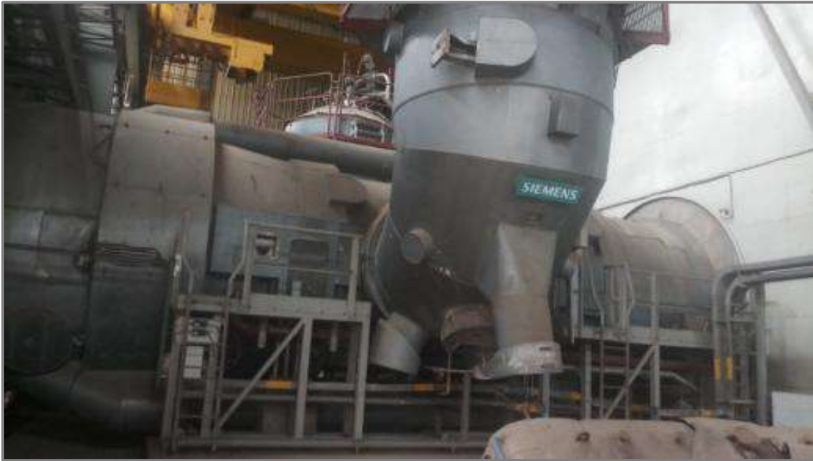
Gas Turbine GT# 1B
