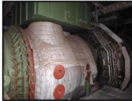
GT-12 Turbine Left View
