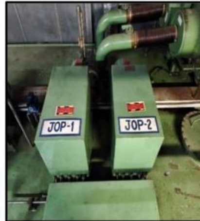
Jockey Oil Pumps – 2nos
