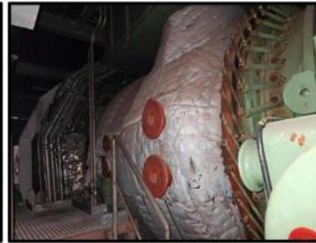
GT-12 Turbine Right View
