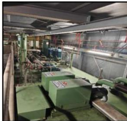
GT - 11 Lube oil skid
