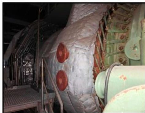
GT-11 Turbine Left View
