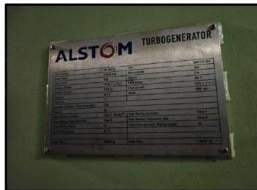
GT-12 Generator Name Plate
