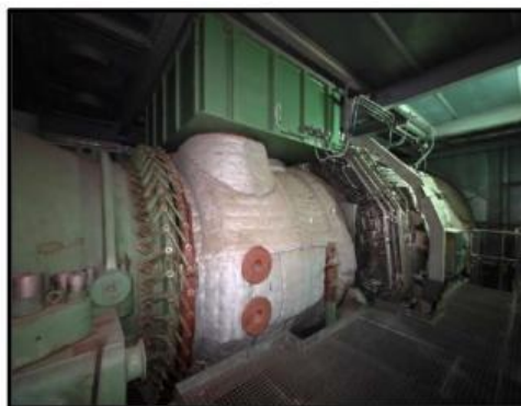
GT-11 Turbine Right View
