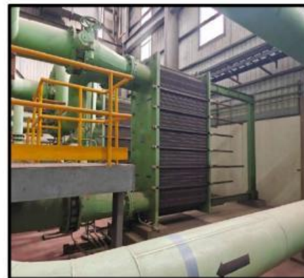
CCW Heat Exchanger-1
