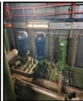
Main Lube Oil Pump -3nos
