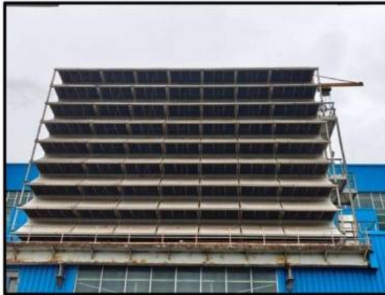
Air Intake System
