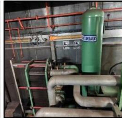
Lube Oil Accumulator
