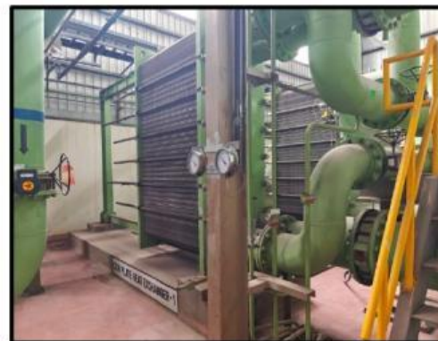
CCW Heat Exchanger-2
