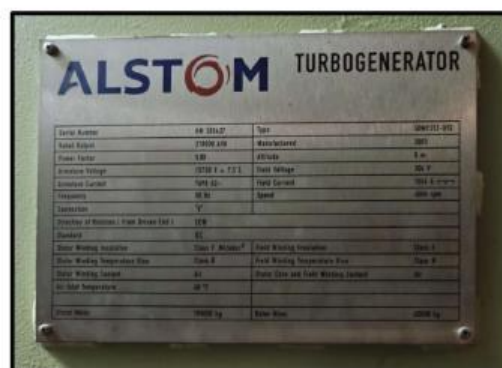
GT-11 Generator Name Plate
