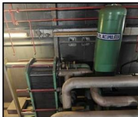
Lube Oil Accumulator
