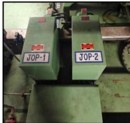
Jockey Oil Pumps – 2nos
