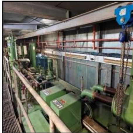
GT - 12 Lube oil skid
