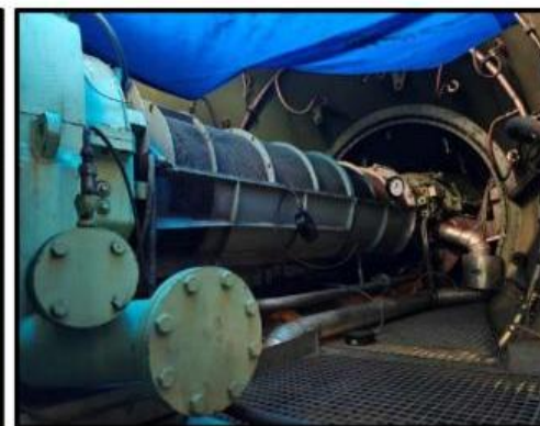
GT-12 Generator and Turbine Coupling
