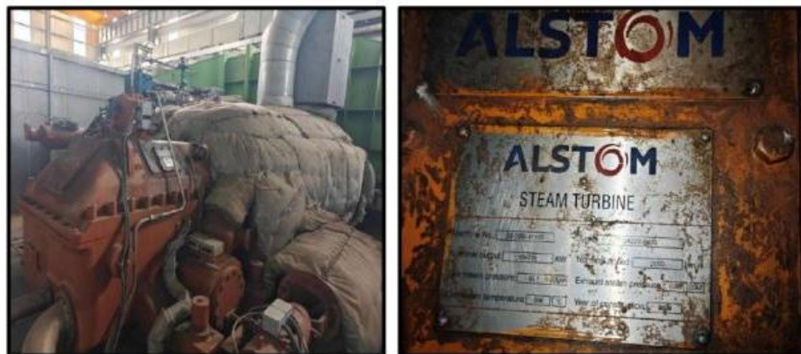
STG LP Turbine & Name Plate
