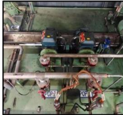
Power Oil Pump – 2nos
