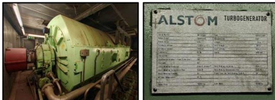
STG Generator & Name Plate
