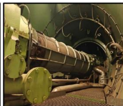
GT-11 Generator and Turbine Coupling
