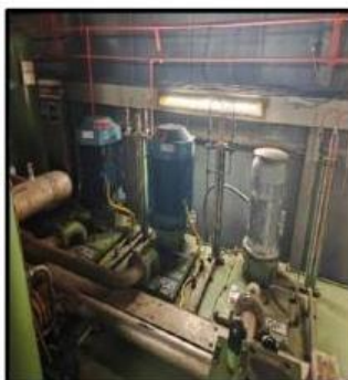
Main Lube Oil Pump -3nos
