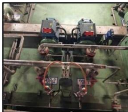
Power Oil Pump – 2nos
