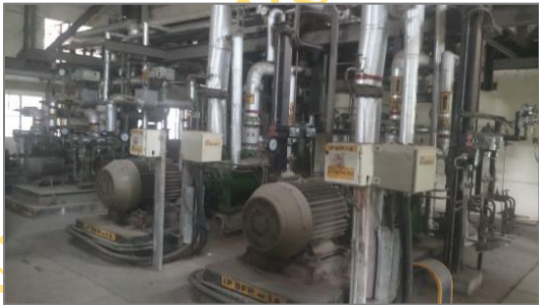
Condition of IP Boiler Feed Pumps
