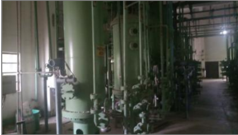
DM Water Plant
