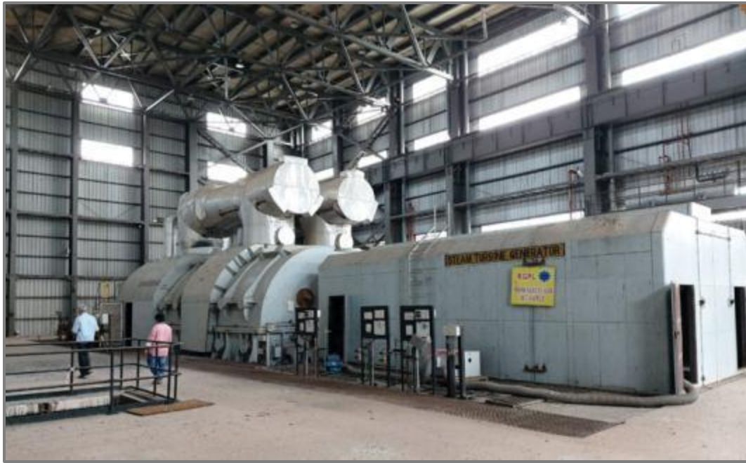
Steam Turbine & Generator
