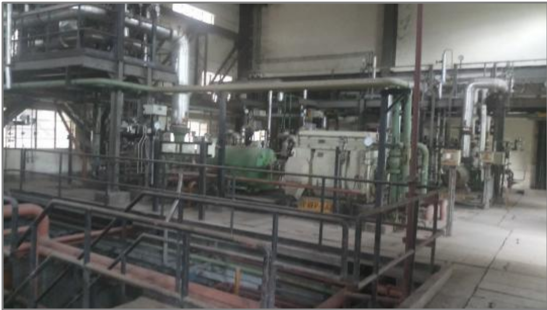
Condition of HP Boiler Feed Pumps
