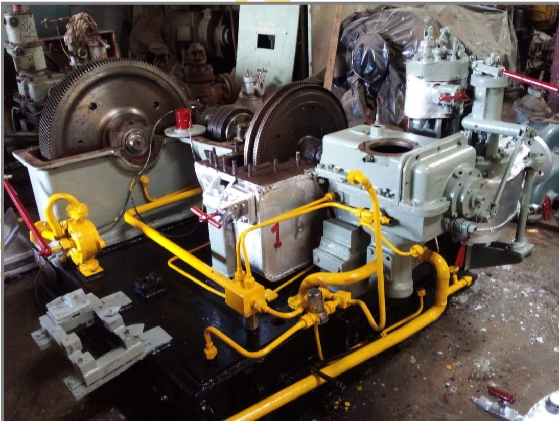
NITIN CORPORATION, 2 Nos.-840 HP each TRIVENI make Steam Turbines MUMBAI.
