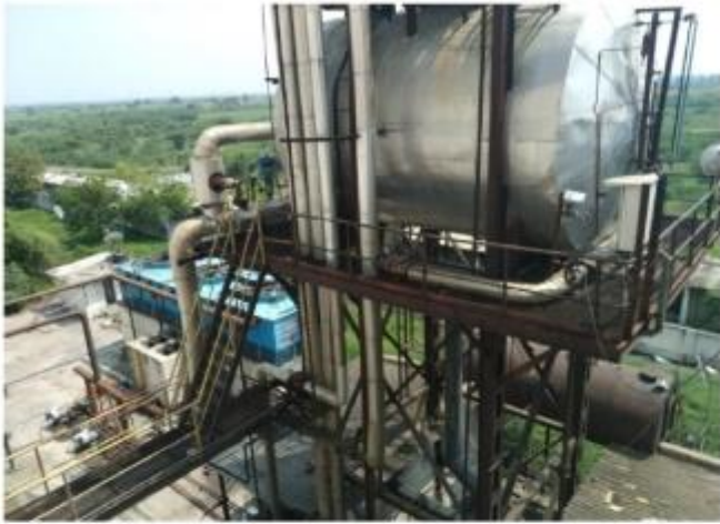
Deaerator & Cooling Tower
