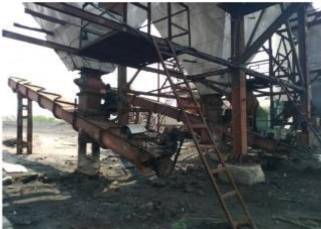
Screw Conveyor in ESP
