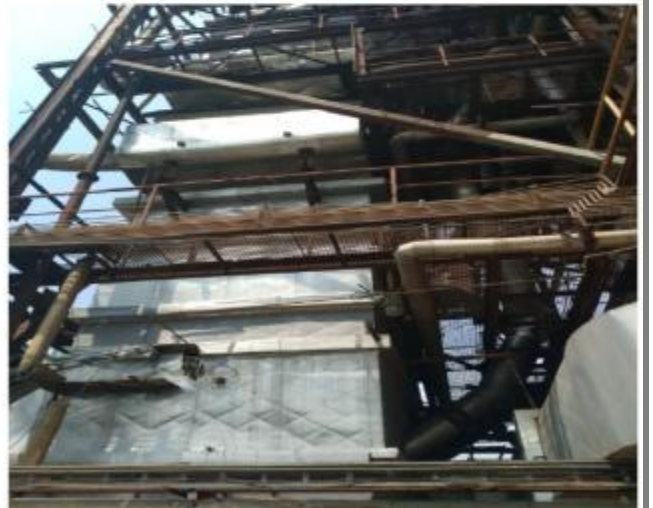
Boiler Second Pass
