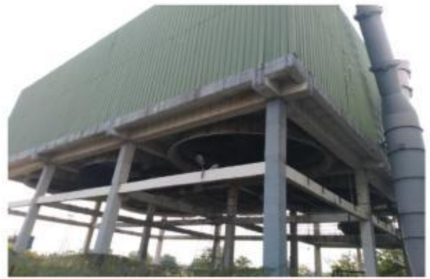
Air Cooled Condenser
