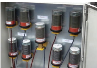
Food waste processing industry: cabinet of Memolubs for the lubrication of bearings and casing of a rotation fermenter.
