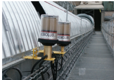
Mineral industry: lubrication of conveyor belt bearings.
