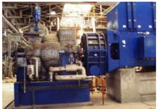
1 No. 10.85 MW Blohm & Voss (2002) make Condensing Type STG Set.
